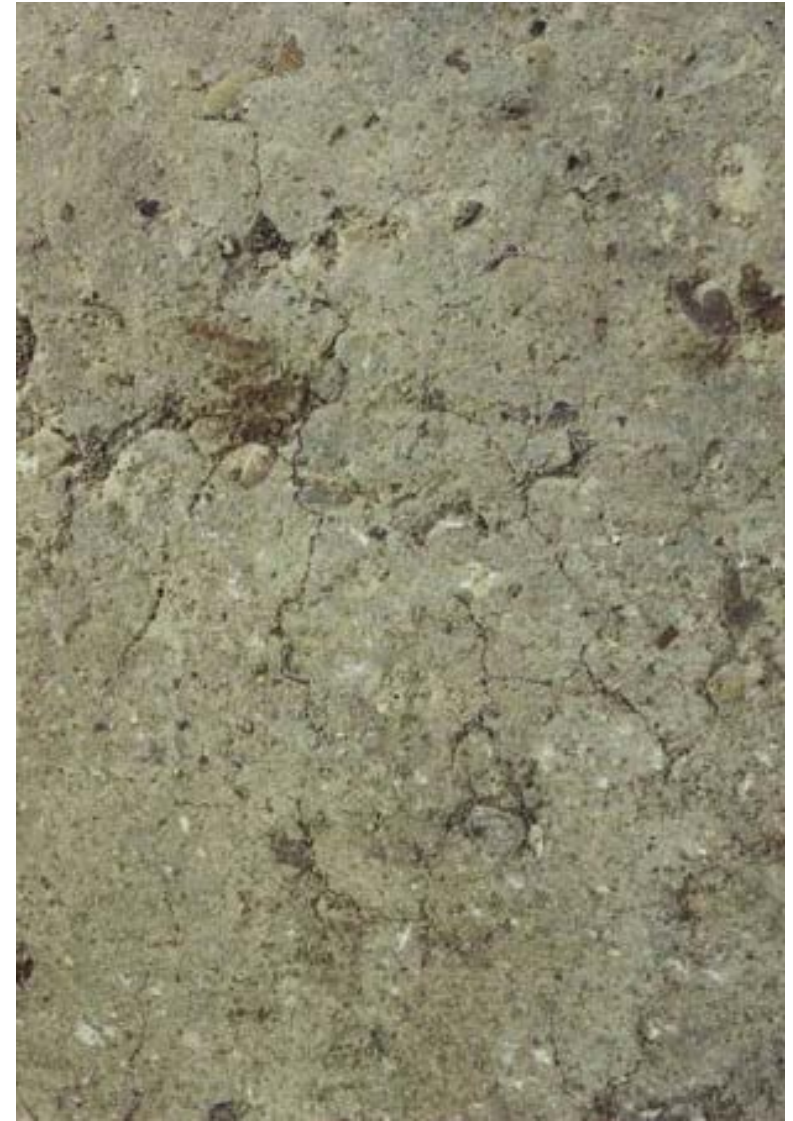
Cracks after Microcracking
