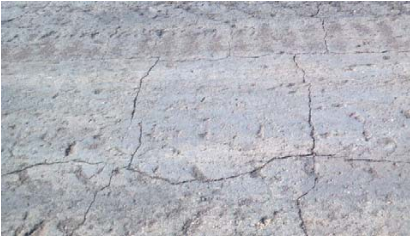
Cracks without Microcracking
